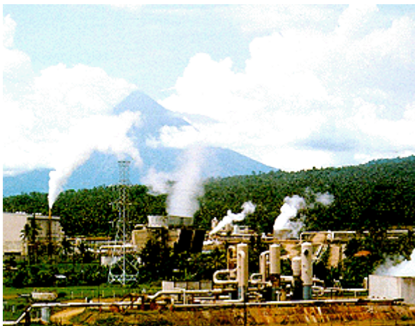
The 289-MW Tiwi complex in Albay
